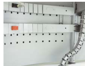
Power and communication wires travel up and down, from one side to another, hidden in large gutters.
